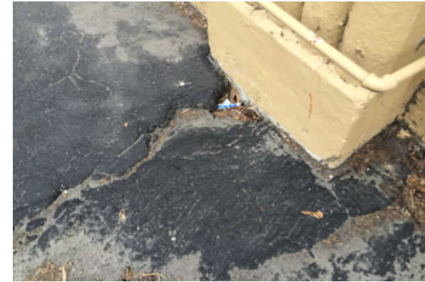
AC paving is cracking which can cause water infiltration
