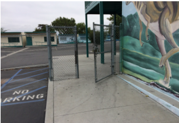
ADA parking stalls and path of travel are not compliant
