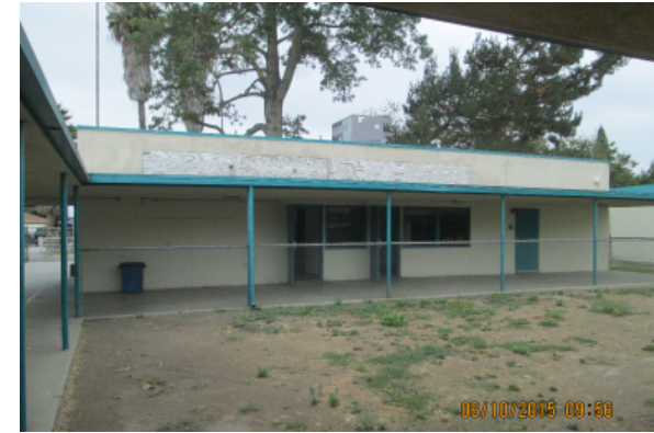
Wood and paint is peeling and deteriorating
