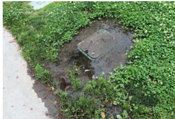
Irrigation system is inoperable
