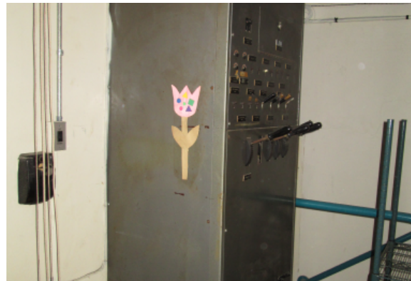
Old distribution board needs replacement
