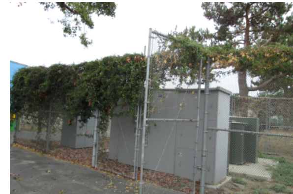
Lack of distribution system maintenance
