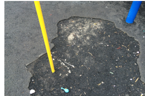
Play surface is degrading
