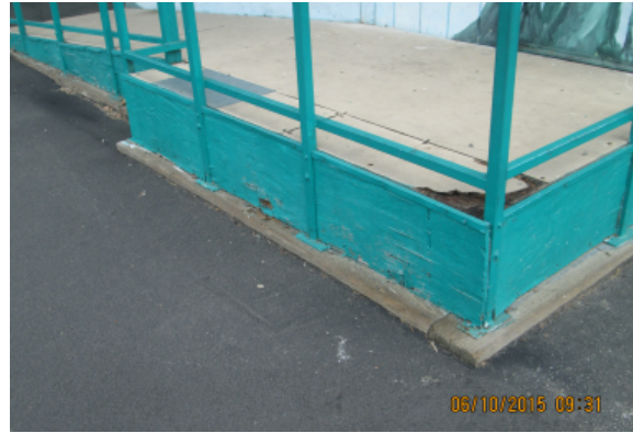
Wood and paint is peeling and deteriorating
