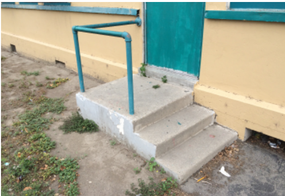
Stair handrails and nosings are missing
