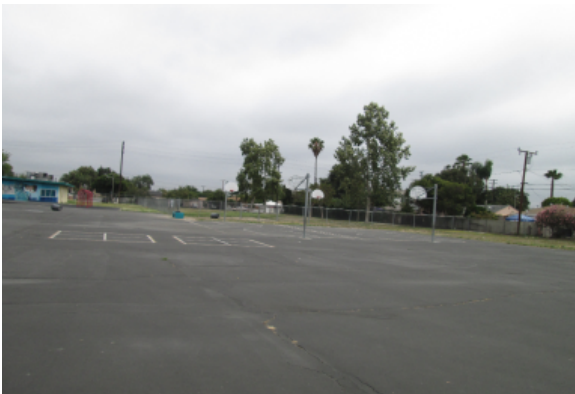
Inadequate site lighting coverage
