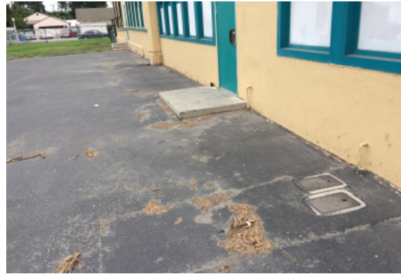
Classroom is not accessible, may require ramp
