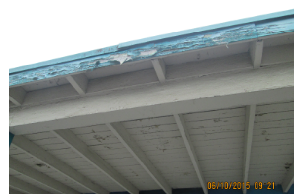
Paint is peeling and cracking at exterior canopy
