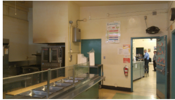
Kitchen equipment does not fit under hood
