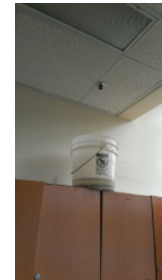
Secondary condensate drain in use
