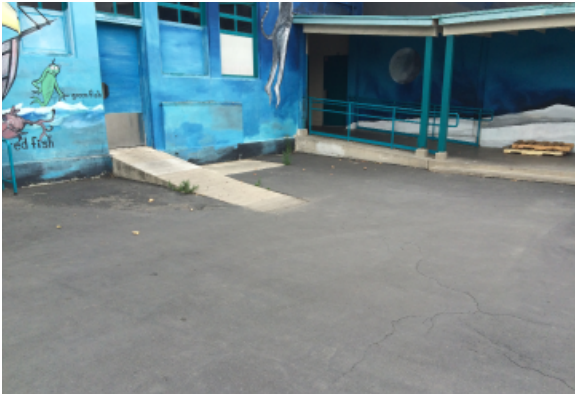
Ramp is not compliant and paving is not flush with walk
