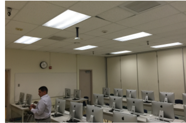
typical overhead supply and return grilles
