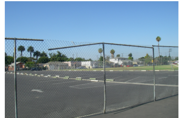
Broken chain link fencing
