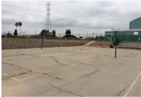
Cracking in pavement
