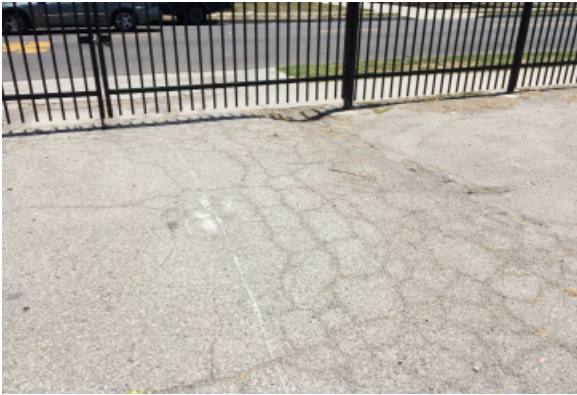
AC paving is cracked/depressed
