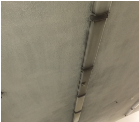
Original surface mounted fixtures are inefficient
