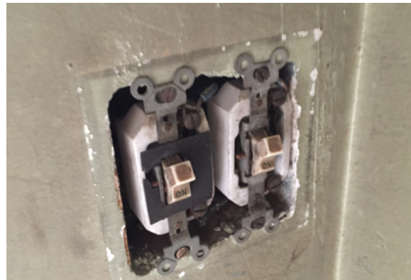
Outlets without protective cover plates
