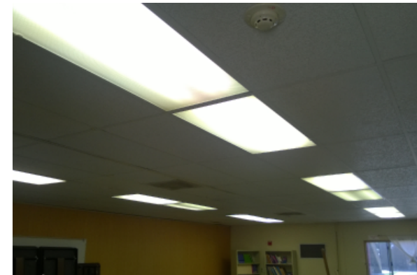
Typical classroom lighting
