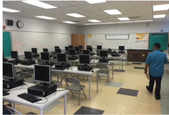
Computer lab with overhead supply and return grilles
