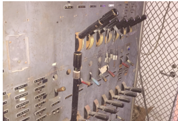
Old distribution equipment needs replacement
