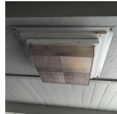
Typical exterior surface mounted light fixture
