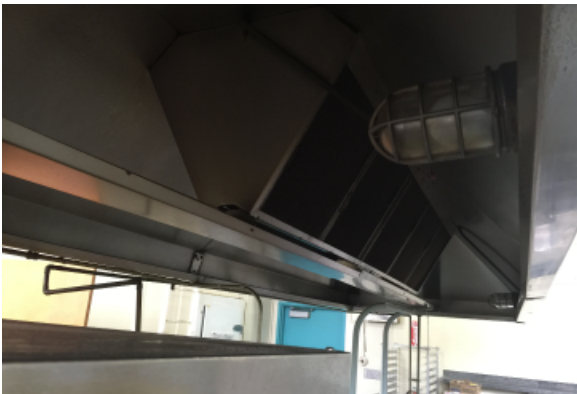
Kitchen hood without fire suppression system
