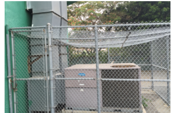
Ground mounted package unit without outside air intake
