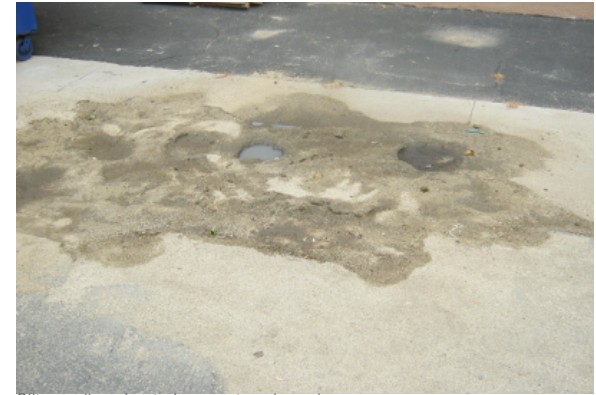
Silt ponding due to low spot and erosion
