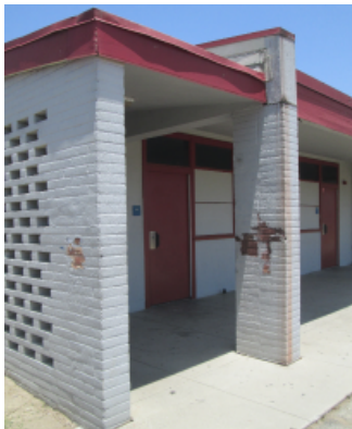
paint is chipping and peeling, metal coping is warped
