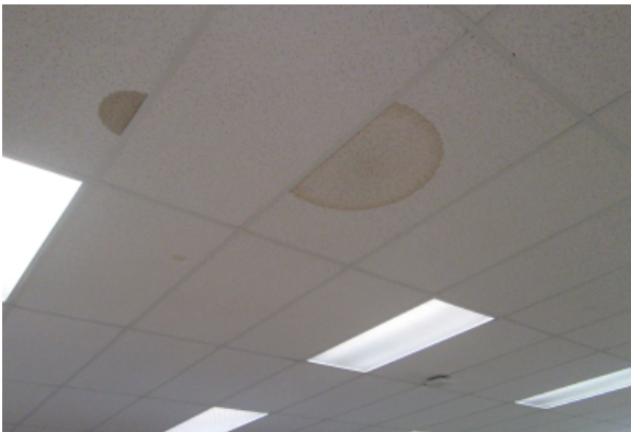
Water damaged ceiling tiles
