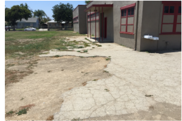
Abcdefg AC paving heavily degraded
