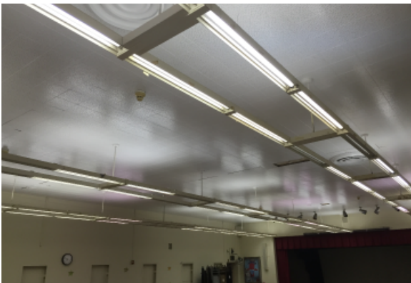
Typical condition of interior pendant light fixtures
