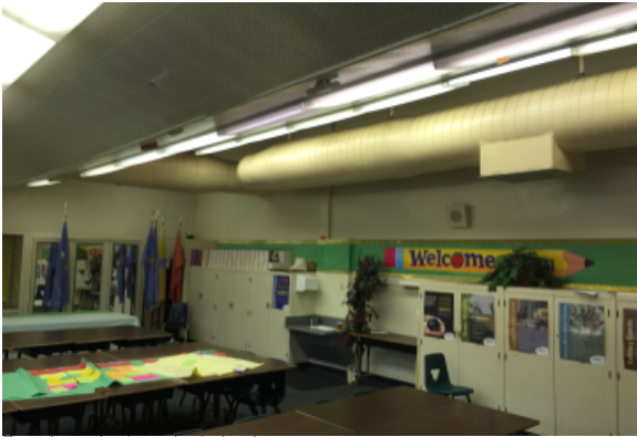
Supply and return ducts in classroom
