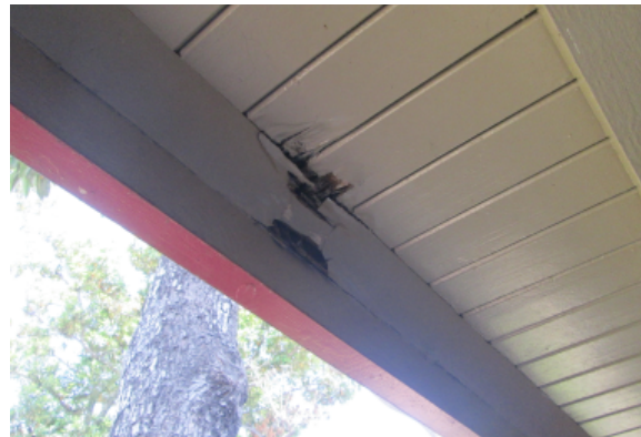
Covered walkway wood deteriorating
