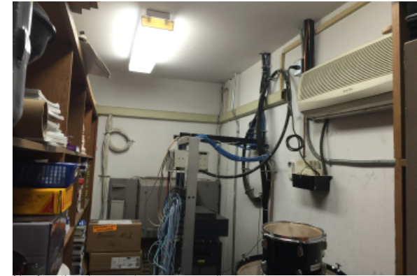
Nonfunctional computer room ac unit
