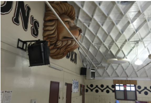
Cafeteria with gas unit heaters no ventilation no AC
