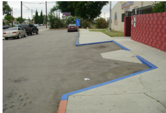
Missing proper drop-off width/length/signage/marking
