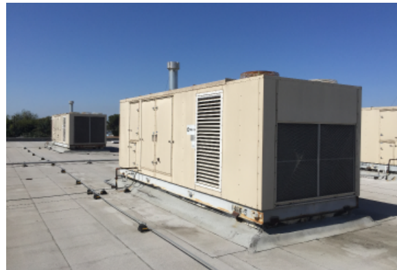
Typical Multi-zone air handler
