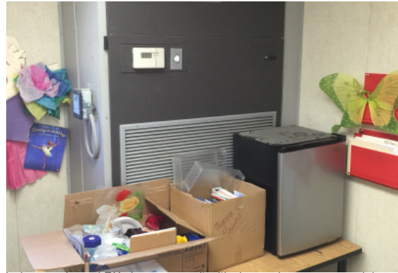
Indoor packaged DX classroom unit with demand response module
