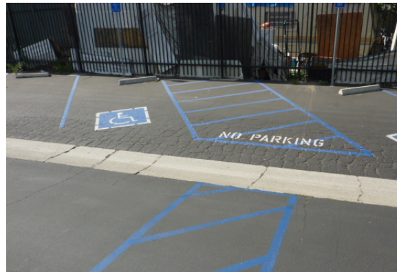
Non-compliant ADA parking on south side of site
