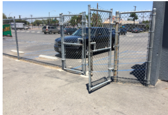
Gate hardware and width is not compliant
