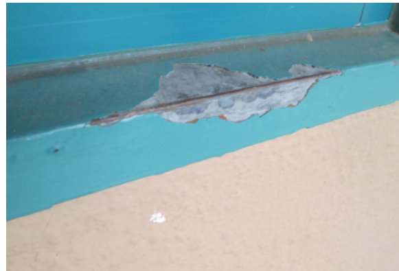
Paint peeling on window frames
