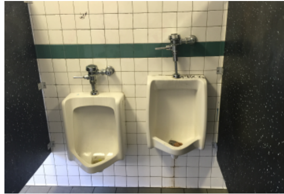
Damaged urinal piping
