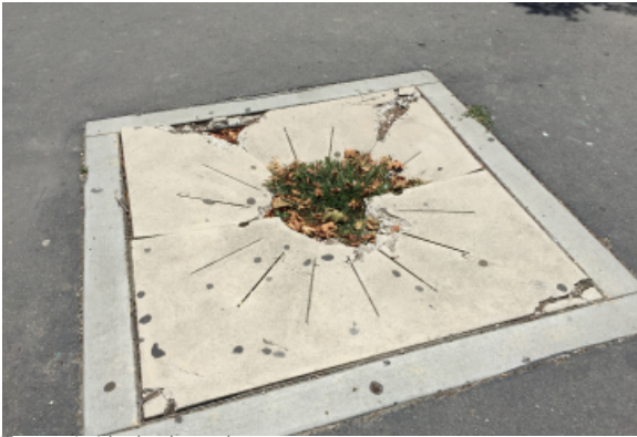
Tree grate tripping hazard
