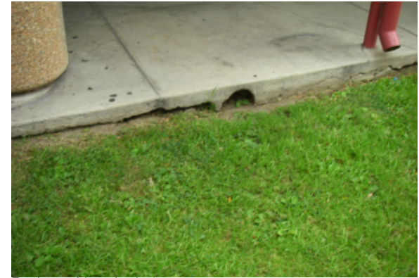
Erosion problems in planter
