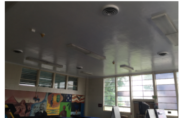
MPR/cafeteria with air conditioning
