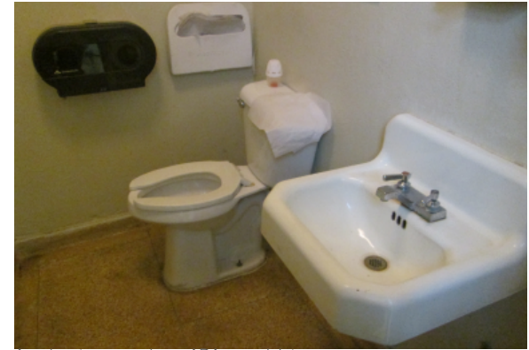
Aged restroom and non ADA complaint
