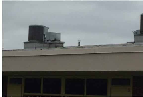
Roof mount CU, OA intake and Flue
