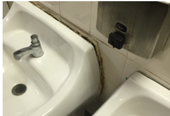
Lavatory separated from the wall
