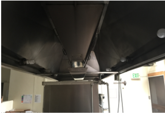
Kitchen hood without suppression system
