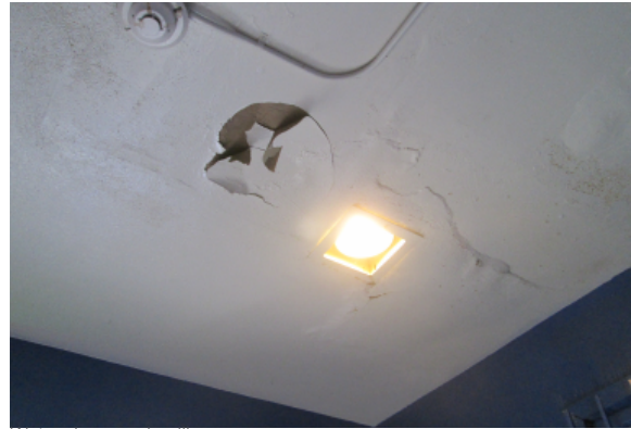
Water damaged ceiling
