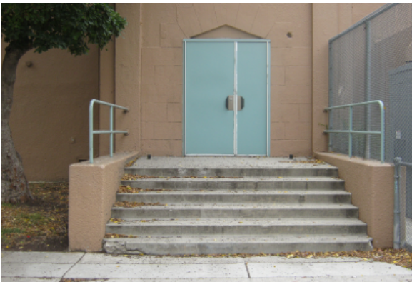
Handrails missing & guardrails non-compliant
