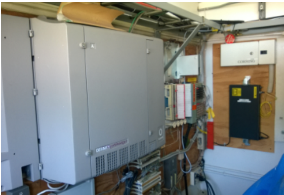
telephone head-in equipment
