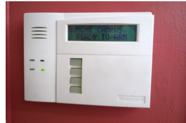
Building access key pad
