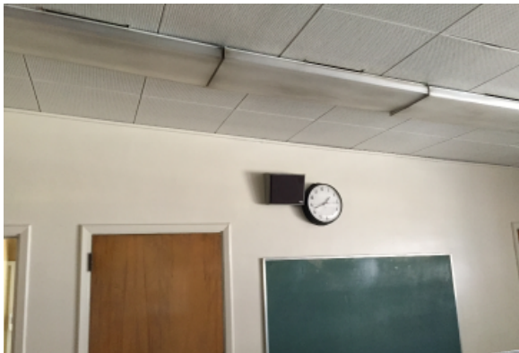
Original classroom lighting
