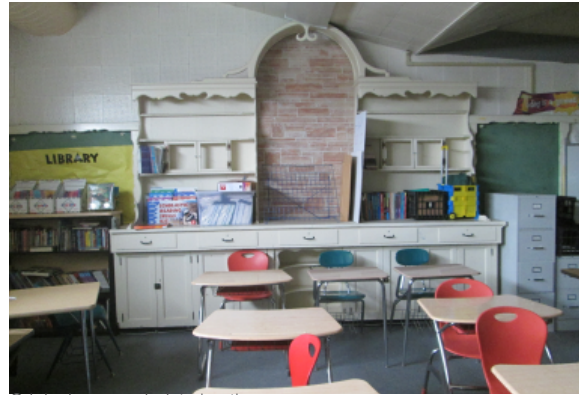
Original casework deteriorating
