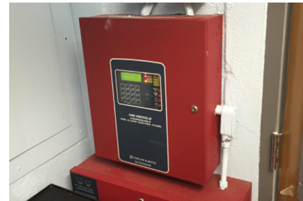
Fire alarm control panel is not up to standards
