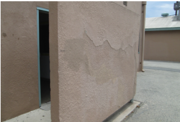
Damaged plaster wall
