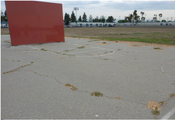
Degrade asphalt on playground
