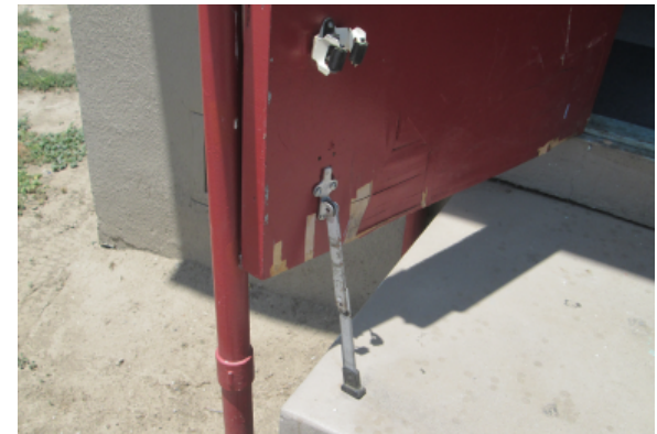
Door damaged and not accessible
