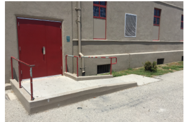
Handrails are missing
