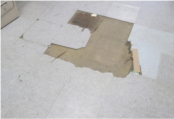
Damaged VCT flooring
