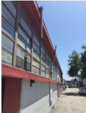
Disconnected flue piping that discharges above classroom ceilings
