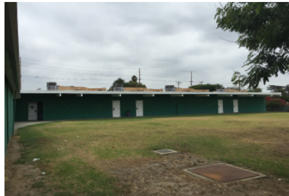
typical rooftop package units
