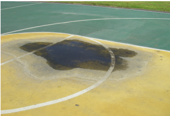
Poor drainage in asphalt paving
