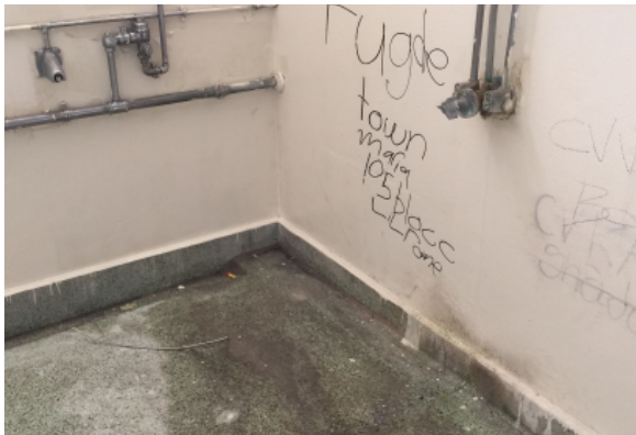
Aged and vandalized showers
