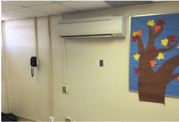
Computer room wall ac unit
