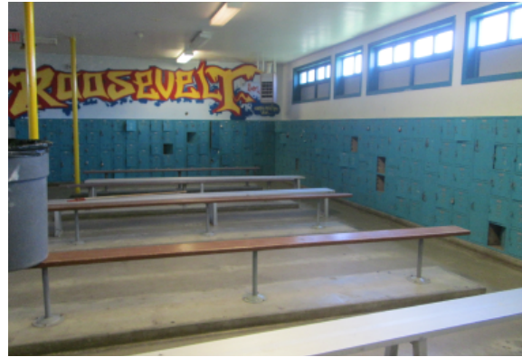
Original lockers deteriorating
