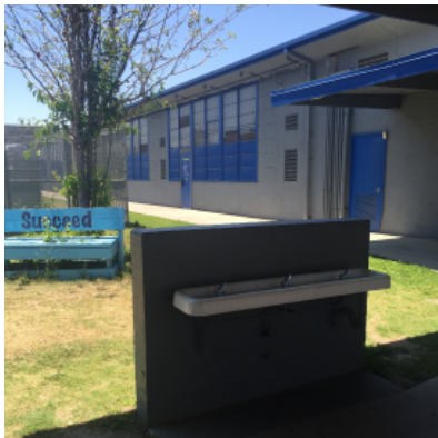
Need to provide accessible drinking fountain and side warning rails
