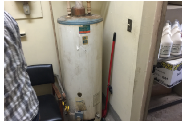
Aged water heater with seismic restraint straps
