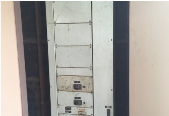
Old switchboard needs replacement
