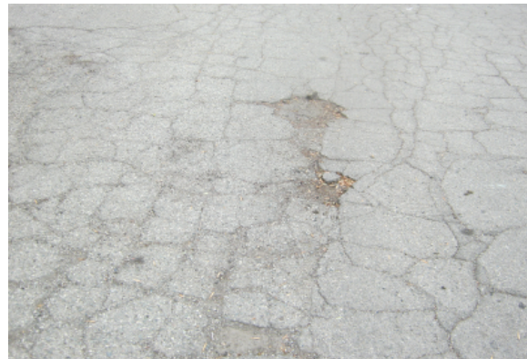
Asphalt cracking allowing for water intrusion
