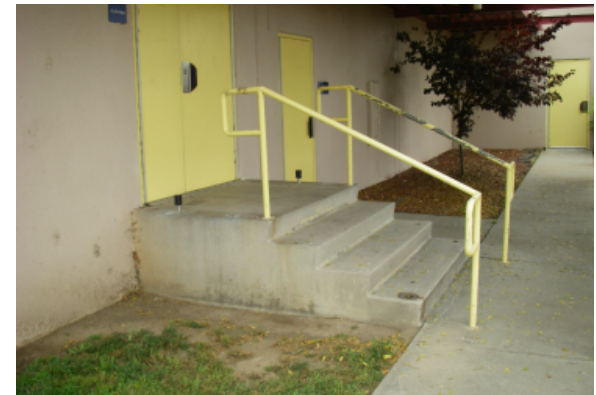
Nosings & landing is non-compliant
