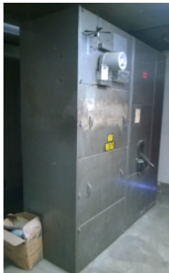
Main switchboard in utility building
