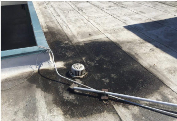
Standing condensate/water on roof
