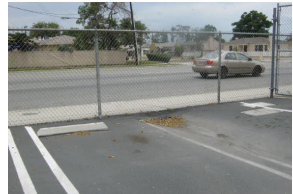
Abcdefg Drain inlet blocked with debris
