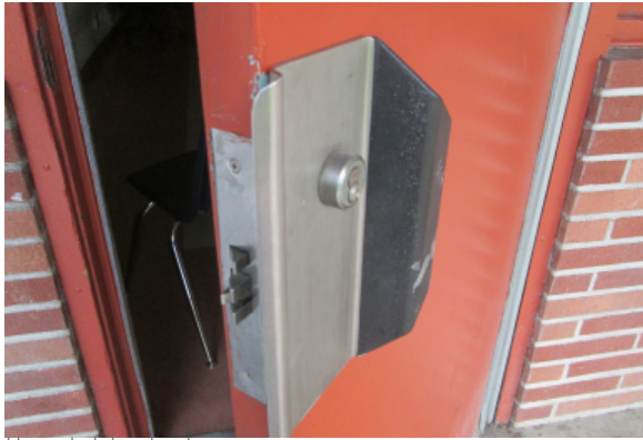
Upgraded door hardware
