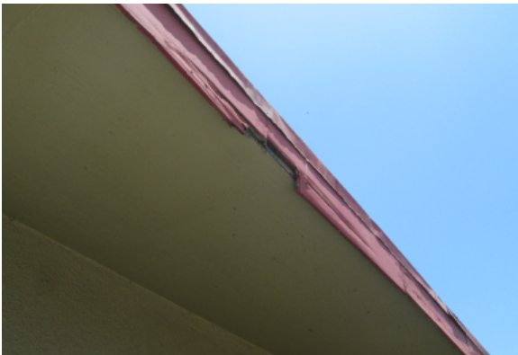
Damaged building fascia
