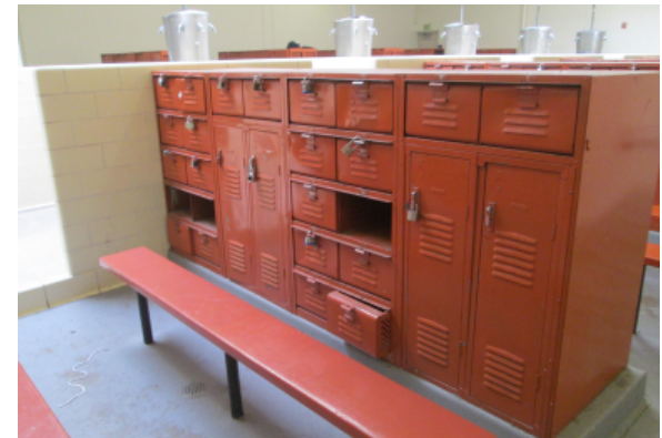
Original lockers deteriorating
