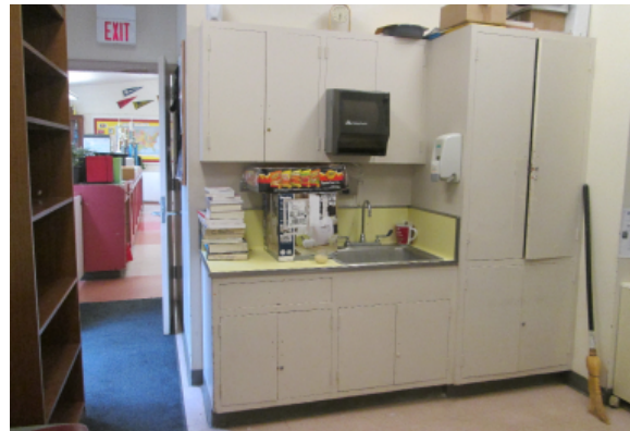
Non-compliant ADA sink
