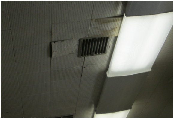
damaged ceiling tiles
