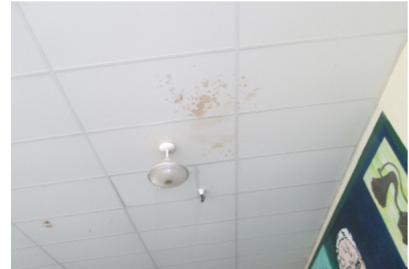
Damage/stains to ACT
