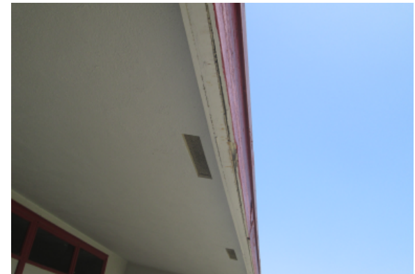
Paint is peeling at fascia
