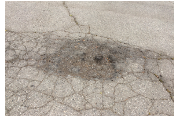
Eroded/cracked asphalt paving
