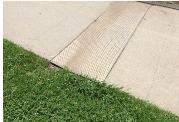
Culvert blocked by landscaping
