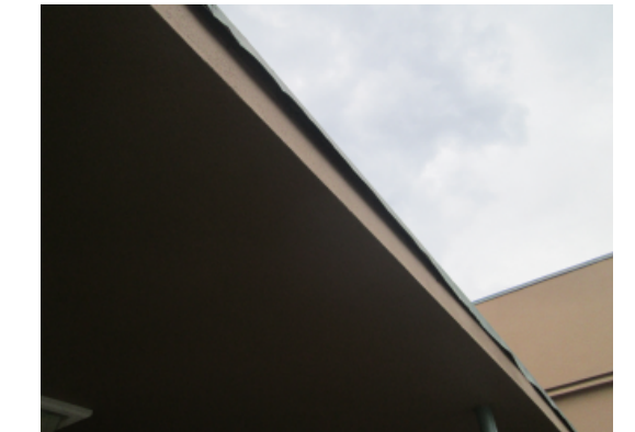
Deteriorating flashing / coping
