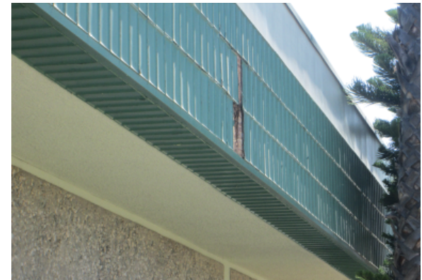
Metal pieces at fascia are missing which can result in water infiltration
