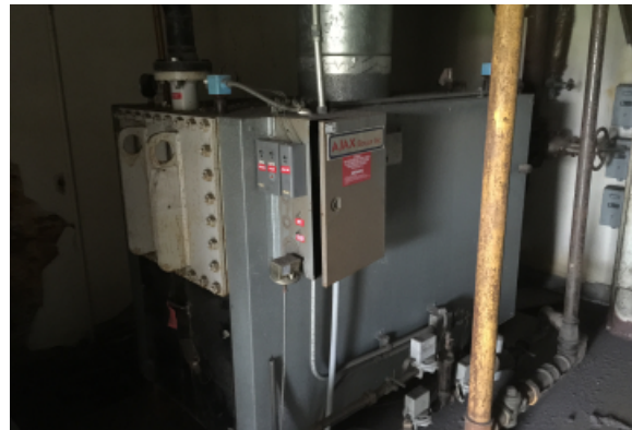
Non-operational domestic water heater
