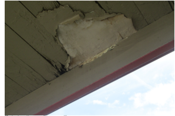
Deteriorating walkway ceiling
