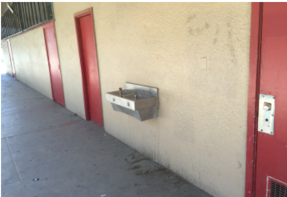
Drinking fountain missing rails
