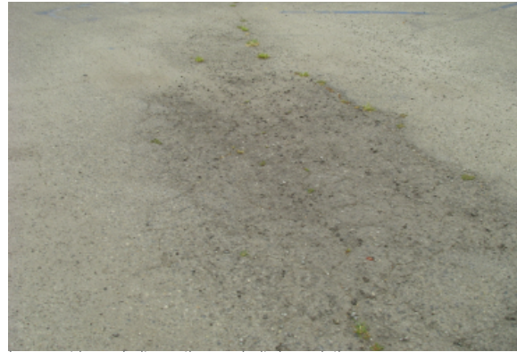
Low spot in asphalt creating asphalt degradation
