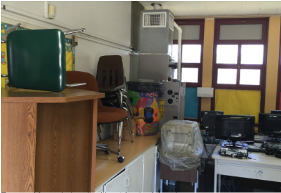
Exposed forced air unit without fresh air input
