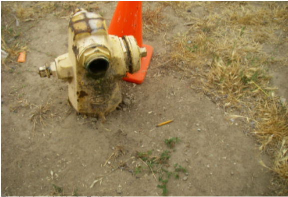
Fire Hydrant buried. Outlet is low.
