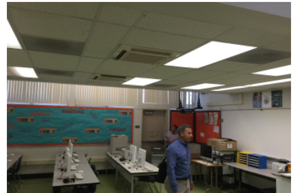
Computer room with Cassette type dx cooling units
