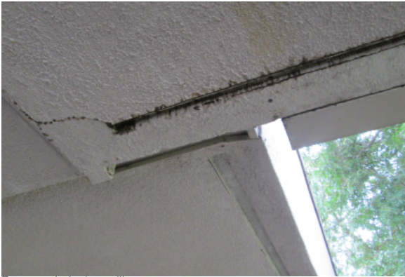
Damaged plaster ceiling
