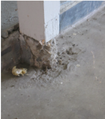
Deteriorating exterior column
