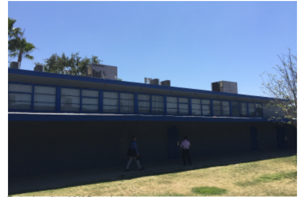
typical rooftop HVAC equipment
