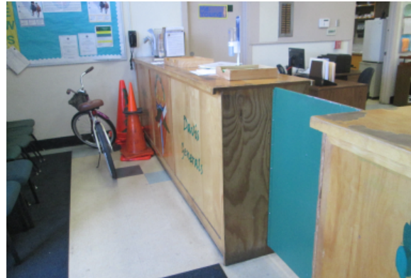
Original reception casework is deteriorating
