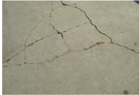
Large cracks in concrete paving
