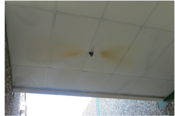
Damage/stains to ACT
