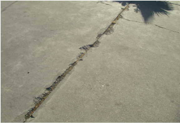
Large chips in concrete paving
