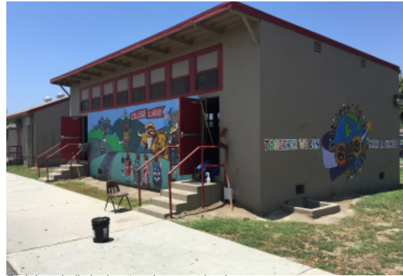
Stair handrails lack extensions, nosing have no grooves nor contrasting color
