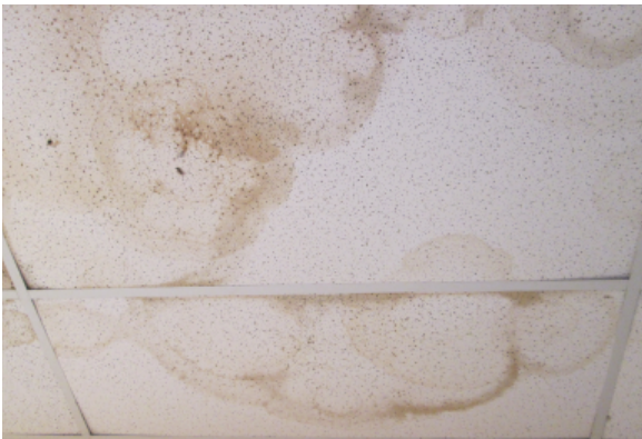
Water damaged ceiling tiles
