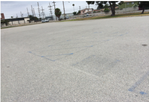
Lacking ADA stall markings/signage/truncated domes
