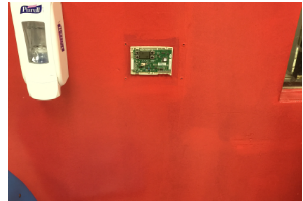
Thermostat missing face plate
