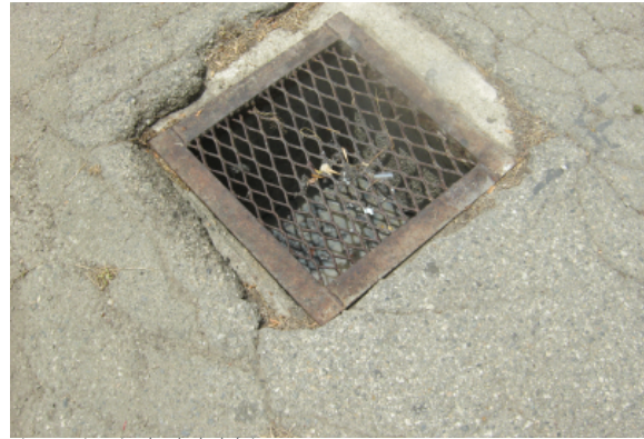
stagnant water in drain inlet
