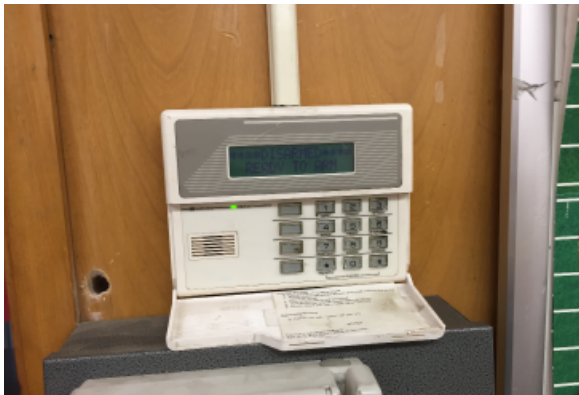
Burglary alarm system is old and needs upgrade
