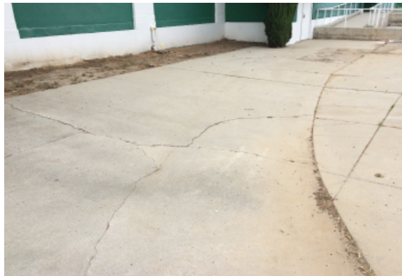
Concrete paving cracking
