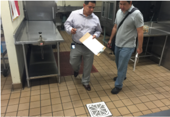
Kitchen floor sink reported to back up on occasion
