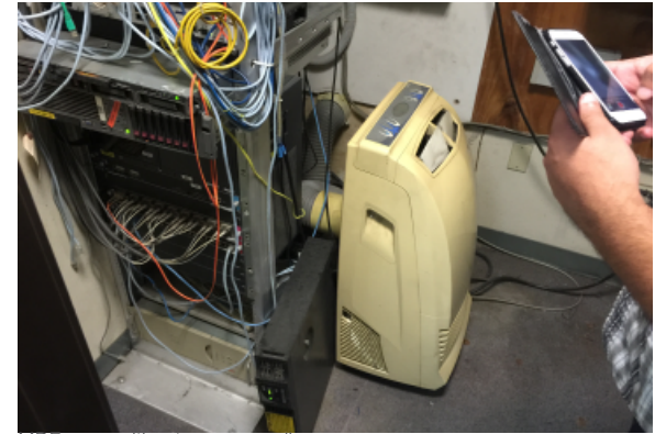
MDF room without proper cooling
