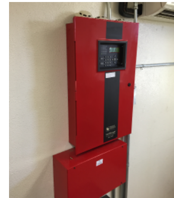
Fire alarm control panel
