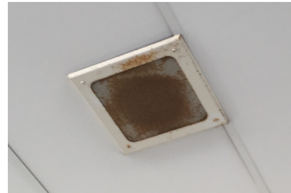
Light fixture is rusting and inoperable
