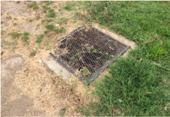
Drain inlet clogged with debris
