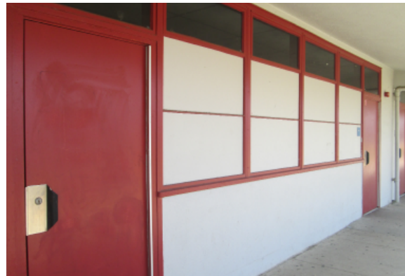
Exterior windows are covered blocking natural daylight
