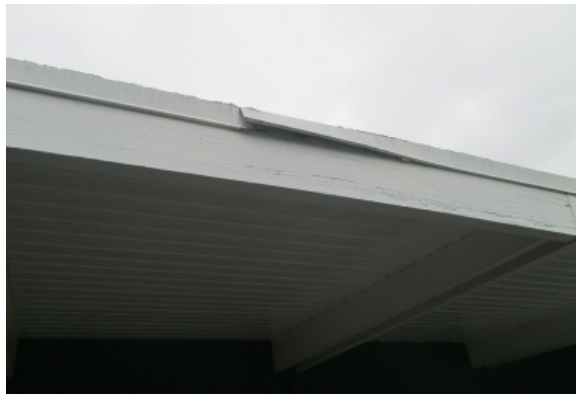
Damaged walkway coping / flashing
