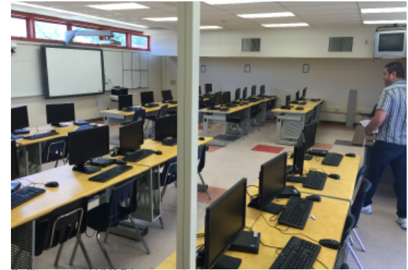
Soffit mounted HVAC in computer lab
