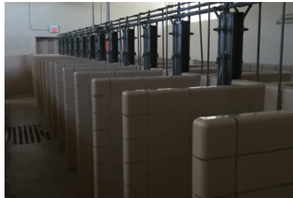
Aged locker showers with galvanized piping
