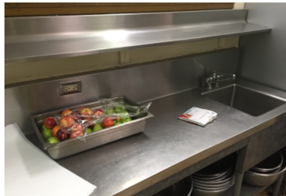
Improper receptacle type used by water sources
