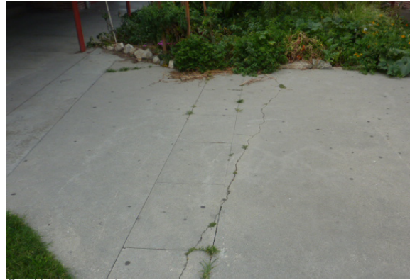
Cracking in concrete
