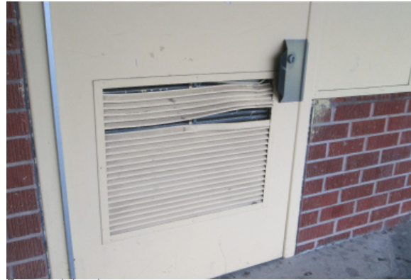
Damaged door louver
