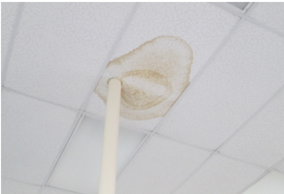
Water damaged ceiling tiles
