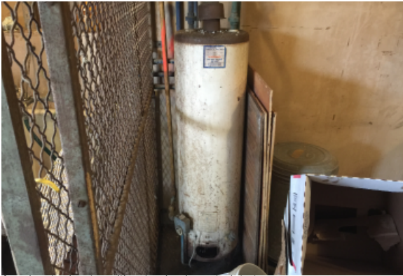
Aged water heater without seismic restraint straps
