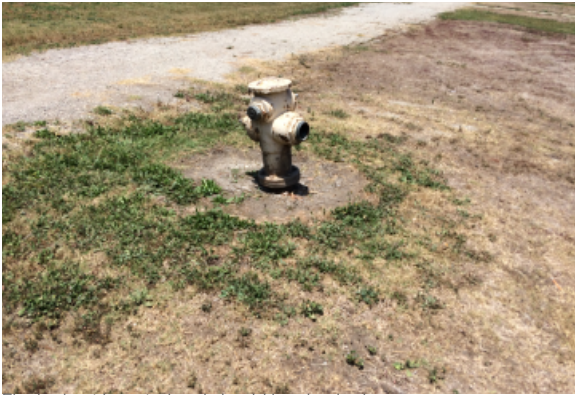
Fire hydrant is rusted and should be checked
