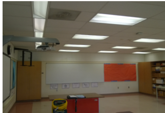
Typical classroom lighting
