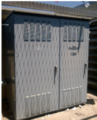
Secondary equipment yard
