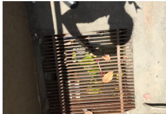
Standing water in drain inlet behind main building
