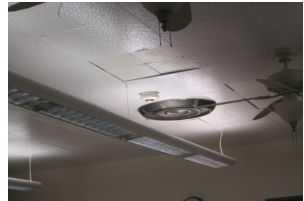
Damaged ceiling tiles
