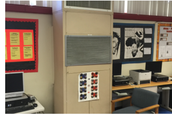
Typical indoor classroom HVAC unit
