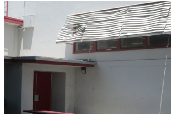
Exterior metal shade damaged
