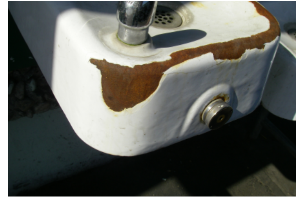
Rusted drinking fountains
