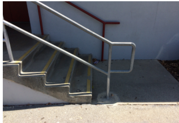
Stair risers and nosing not up to current code
