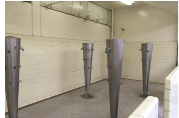
Aged locker room shower
