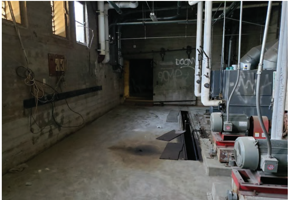
Photograph 18: Section view of AOC2-B1 and B2 in basement of main office building on Compton High School main campus.
