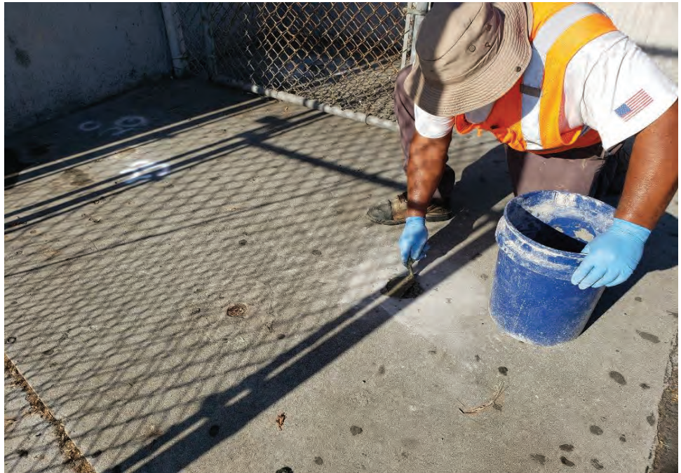
Photograph 16: Worker capping boring with cement to match existing surrounding material on Compton High School main campus.
